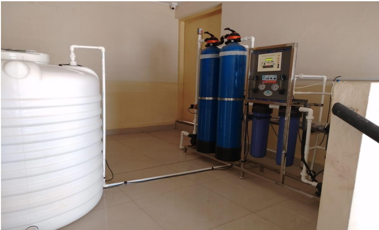
Drinking water facility (RO)
