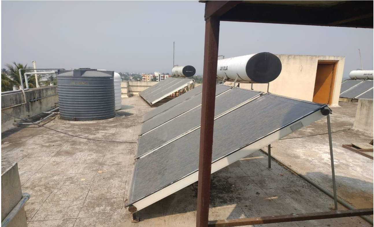
Solar Water Heater
